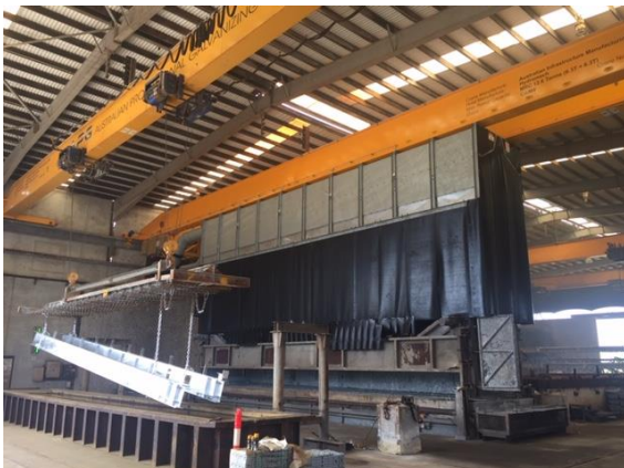
Modern Galvanizing Plant
