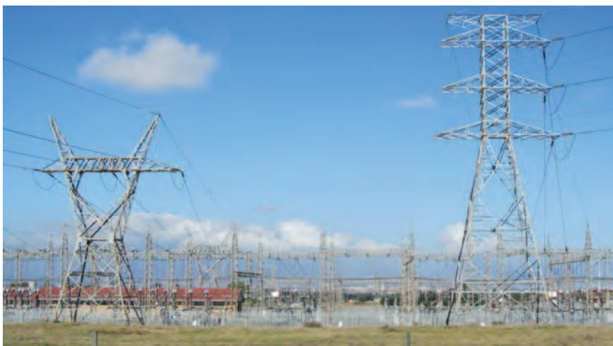
Figure 8: Electrical transmission towers use large numbers of bolted connections for ease of construction and low maintenance in critical infrastructure
