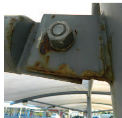
Figure 22: HDG connections can often provide a longer life to first maintenance than painted structures
